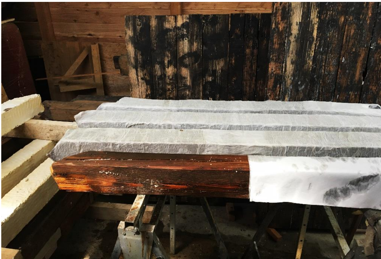
Pic. 5: Compresses on the elements of the wooden barrack B-167. Photo by A.B
