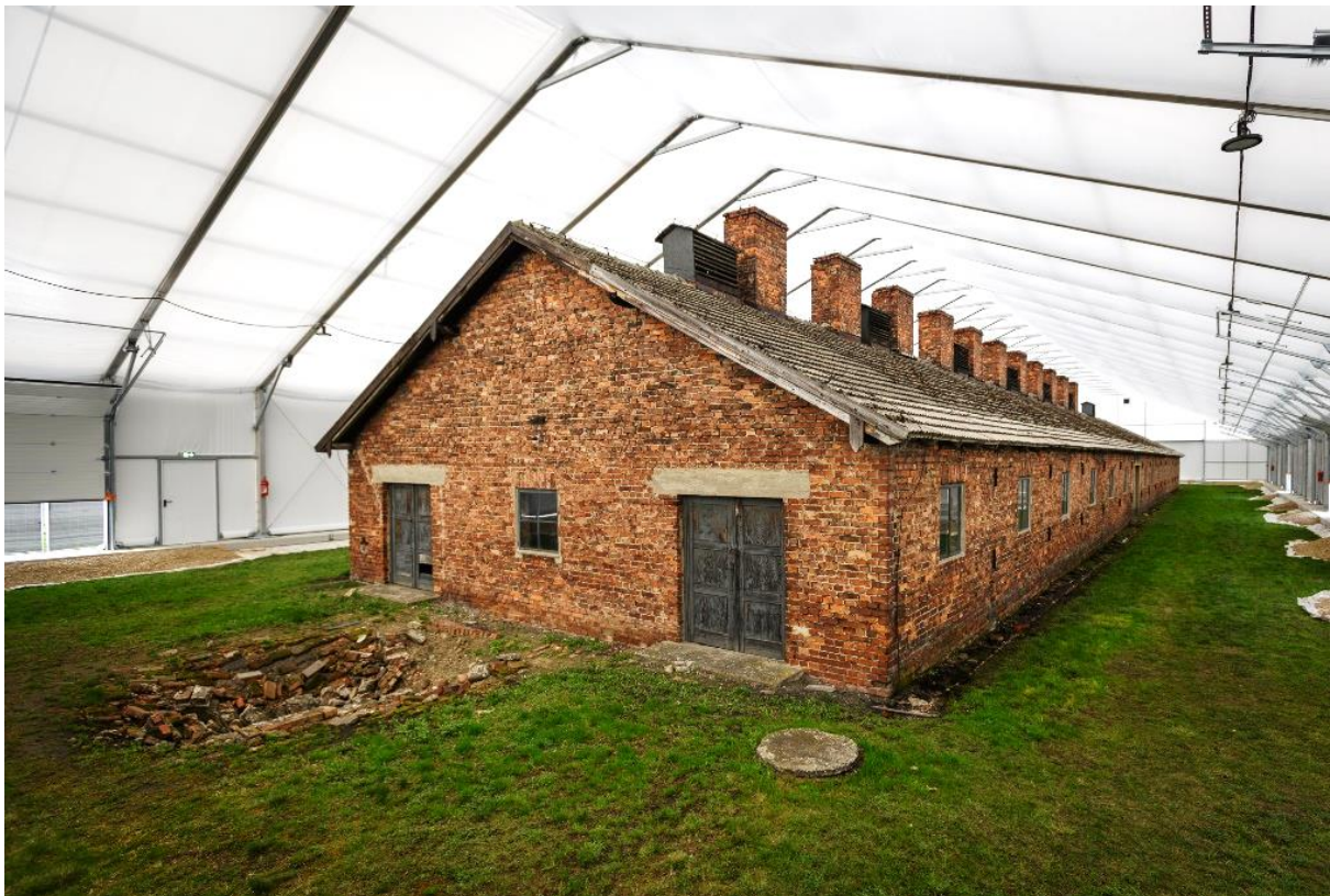
Pic. 3: Assembly of halls over the kitchen and latrine was performed in the spring of 2021. Photo by K. B (ABSM)
