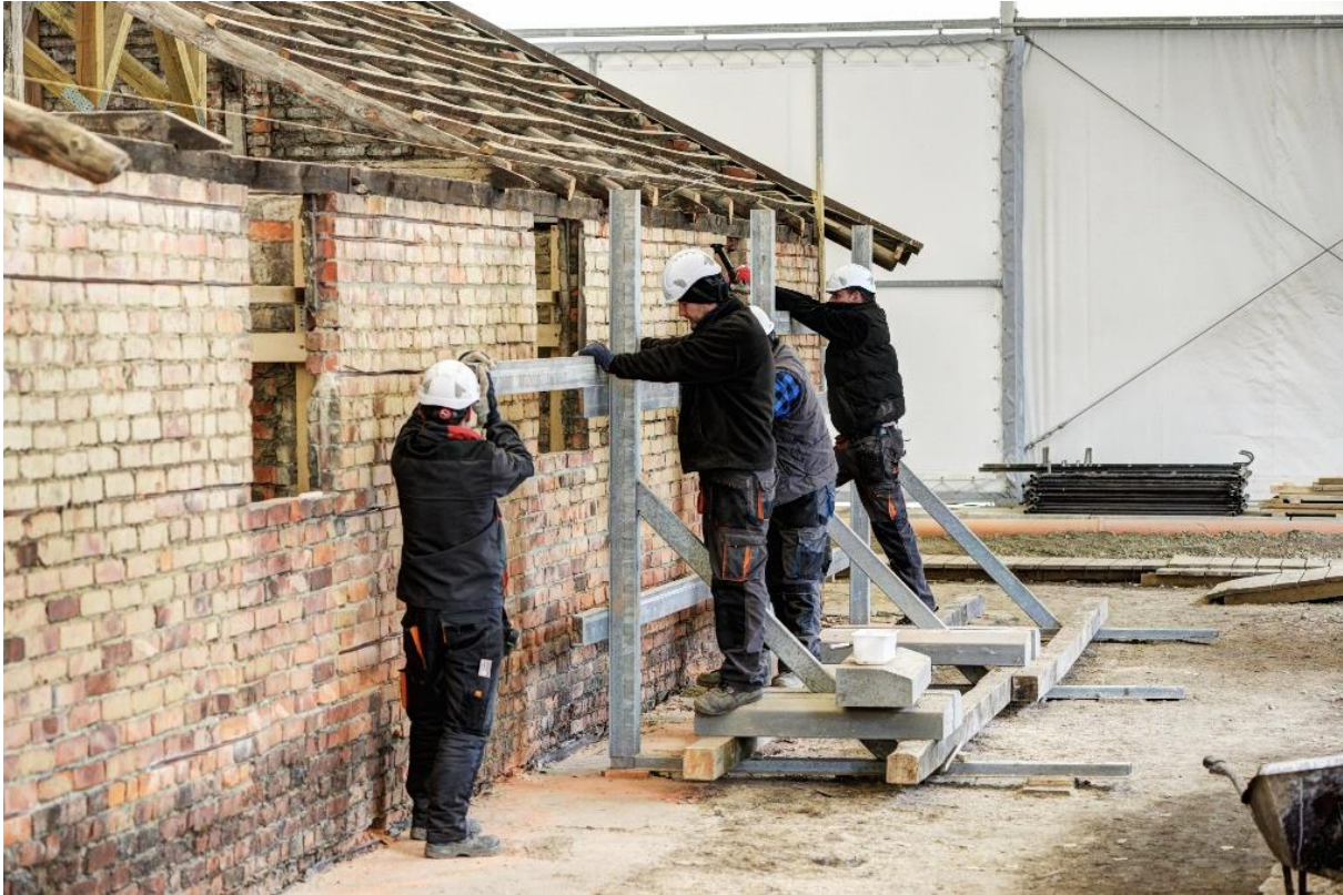
Pic. 4: Strengthening of the barrack B-138 structure, continued in the first half of 202. Photo by K. B. (ABSM)
